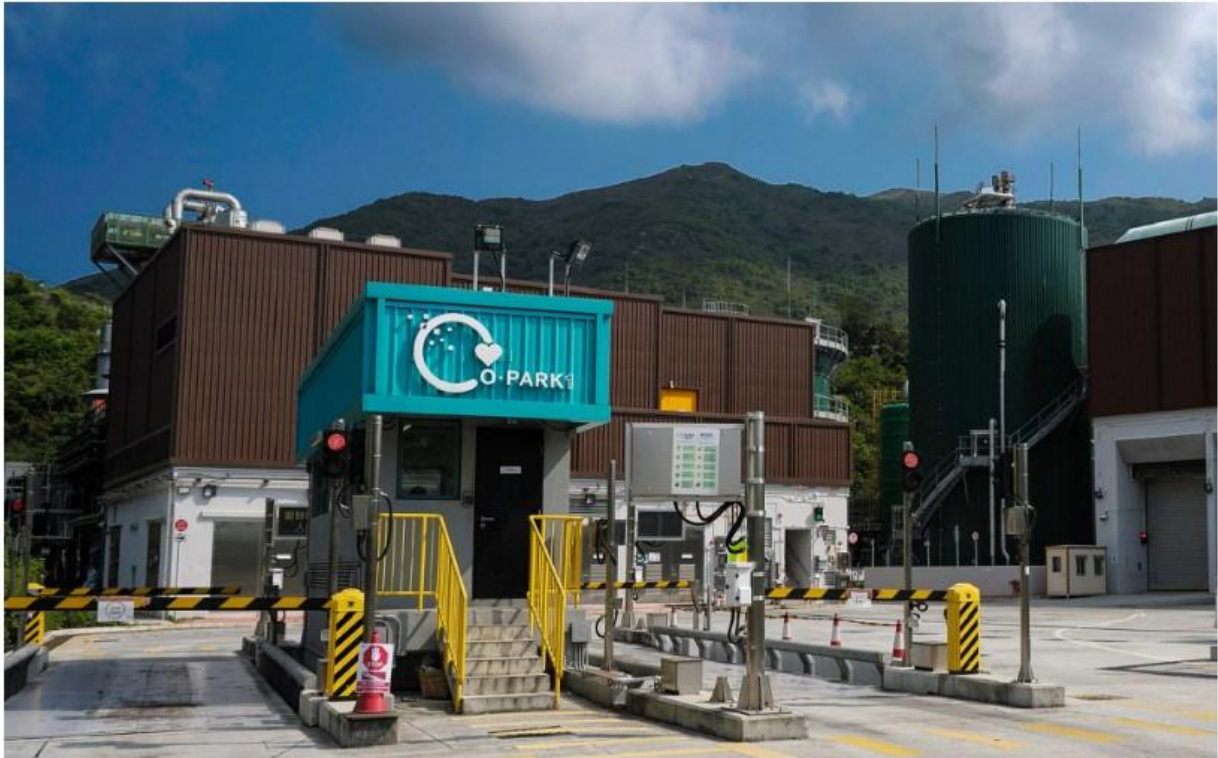
Hong Kong's first organic waste treatment facility, O Park, on Lantau Island, treats 200 tonnes of food waste daily. Photo: hkgbc
